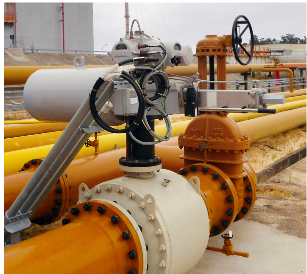
Figure 2. A self-contained electro-hydraulic actuator on a typical tank farm ESD valve installation.
