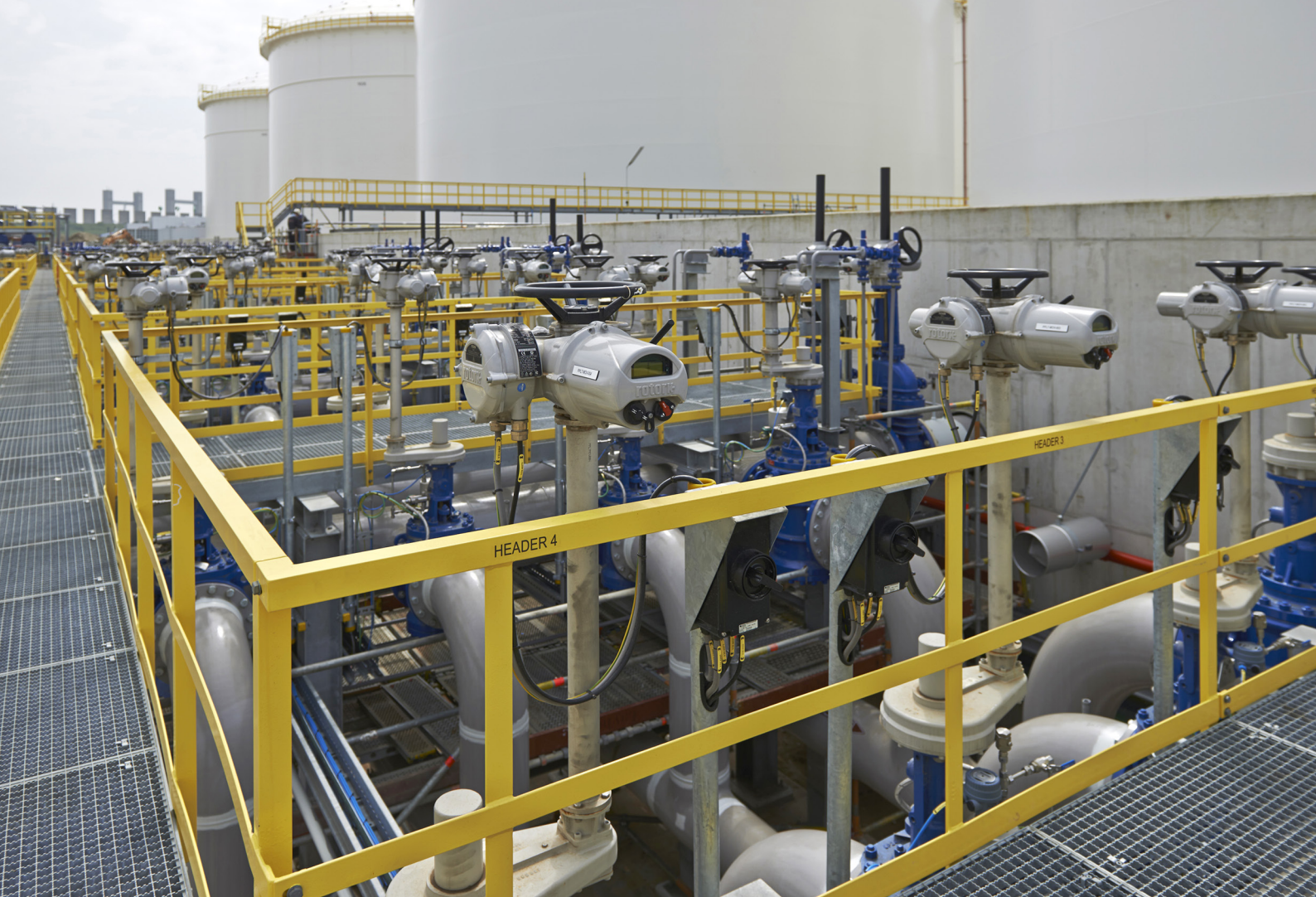
Non-intrusive intelligent electric valve actuators installed on tank farm manifolds.
