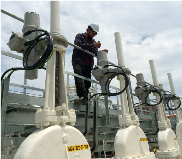
Figure 1. An engineer downloads historical operating data from an actuator using a non-intrusive hand-held setting tool.
