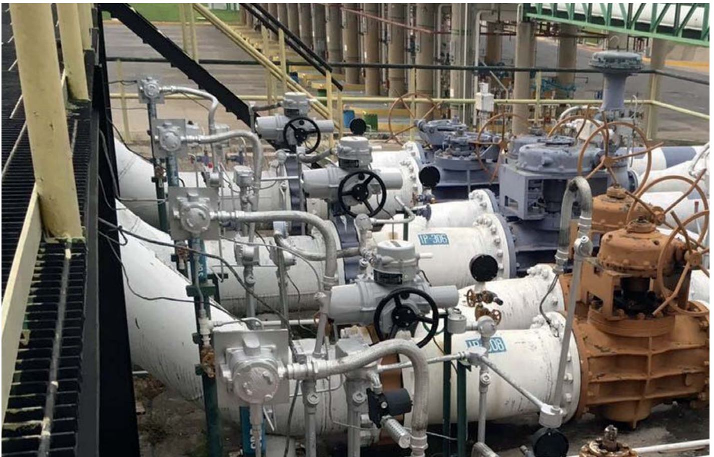
Figure 1: Almost 300 Rotork IQ3 intelligent electric valve actuators now installed in this plant are wirelessly monitored and controlled.
