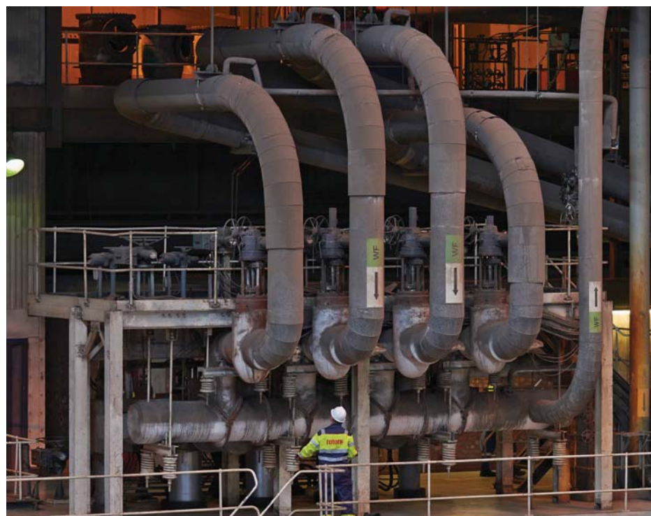
Fig 5 – The ability to objectively analyse information and identify the key areas that are important for each individual site's specific requirements is an essential requirement for effective asset management.
