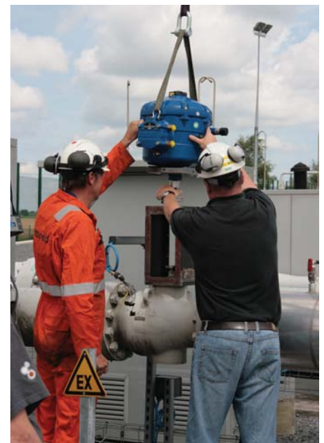
Engineers installing an ATEX certified explosionproof Rotork CVL-5000 actuator at a Fluxys gas blending plant.
