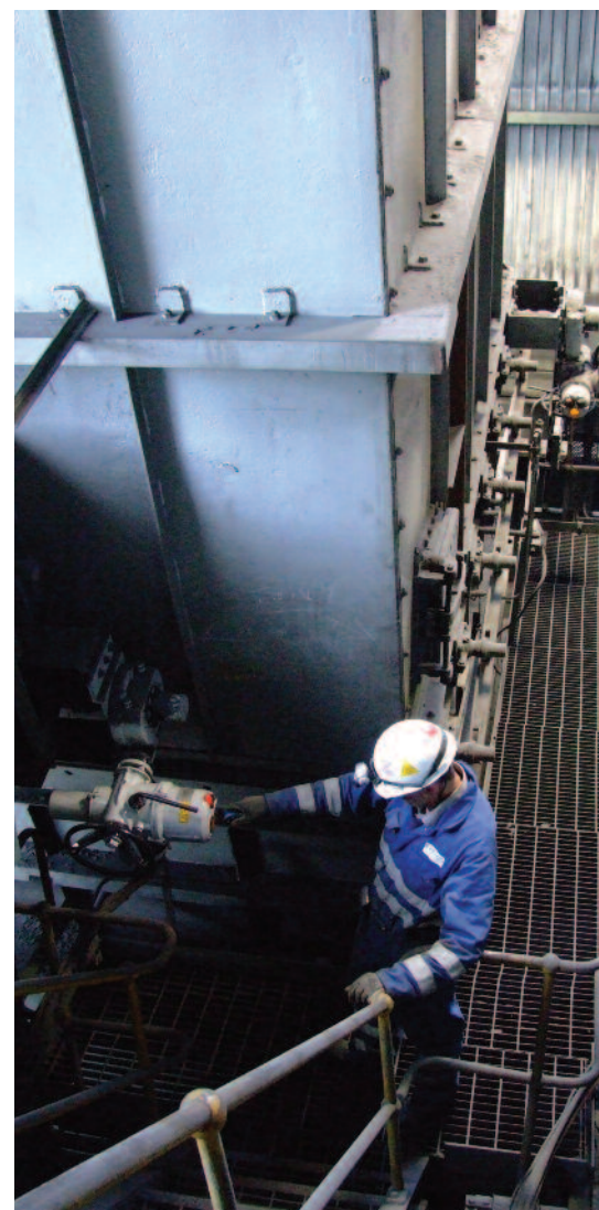
Rotork IQ actuators operating quarter-turn dampers at Aberthaw Power Station.
