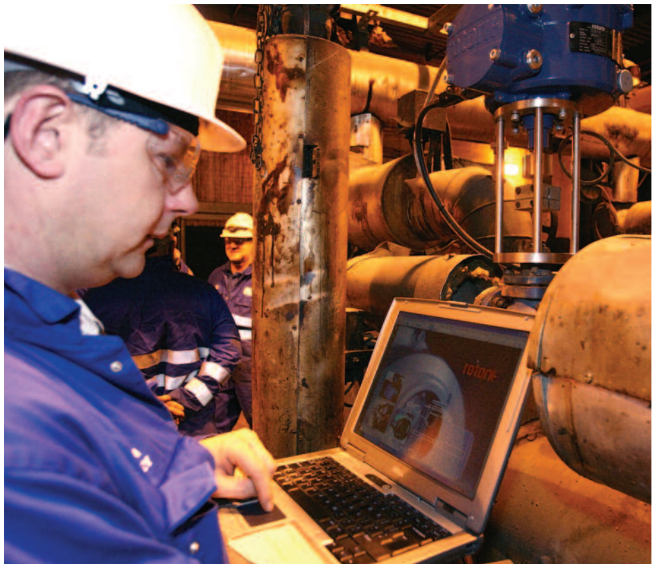
Rotork CVA actuator controlling an inlet regulating steam valve at Drax Power Station.
