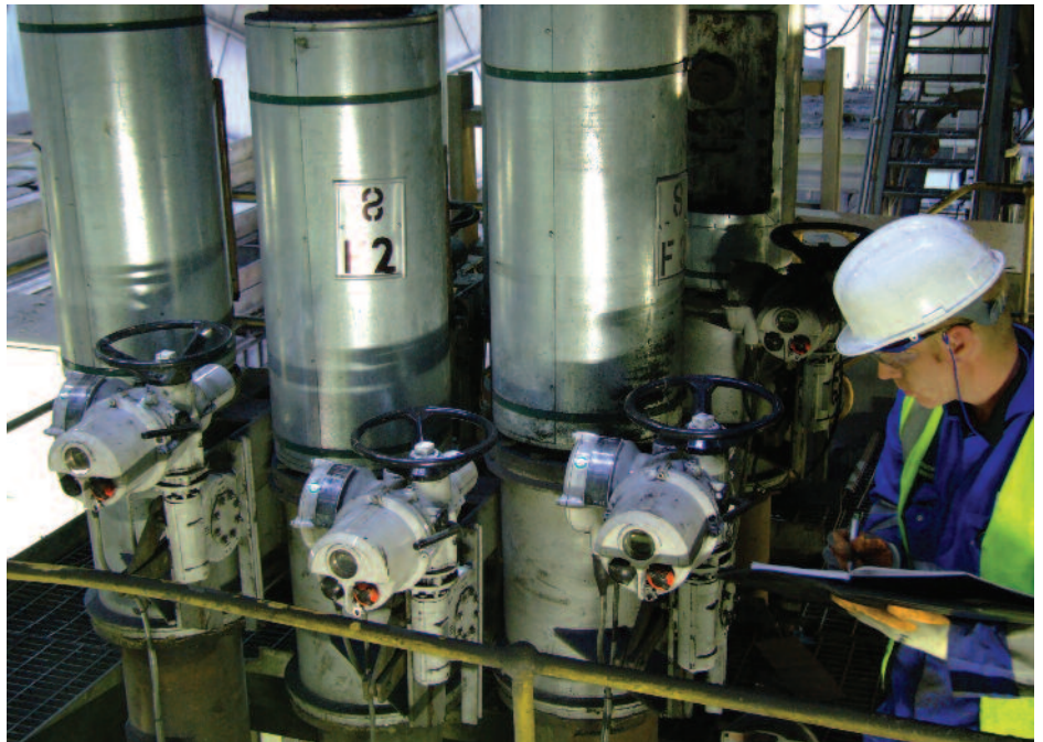
Closely grouped Rotork IQ actuators on quarter-turn air damper duty at Aberthaw Power Station.
