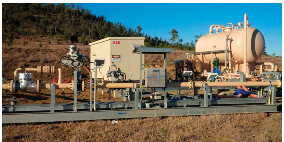
Fig 1: Installation in progress on a typical wellhead and separator skid on the Queensland mainland.
