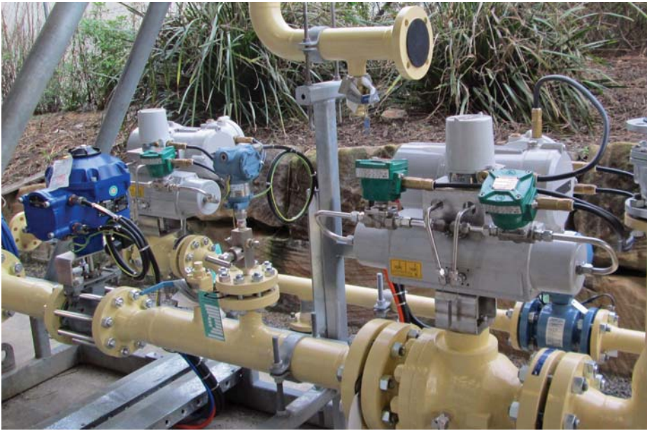
Fig 2: Rotork CVA and Skilmatic actuators installed on a typical Queensland Gas wellhead skid. On the left, a CVA actuator, model CVQ1200, operates a 3 inch (DN80) ball valve to control the gas flow and pressure. Behind the CVA, a Skilmatic Model SI-Q51 electro-hydraulic actuator operates a 2 inch (DN50) safety shut-down ball valve on the water extraction line. The Skilmatic Model SI-Q60 on the right is controlling a 4 inch (DN100) safety shutdown ball valve on the gas line.
