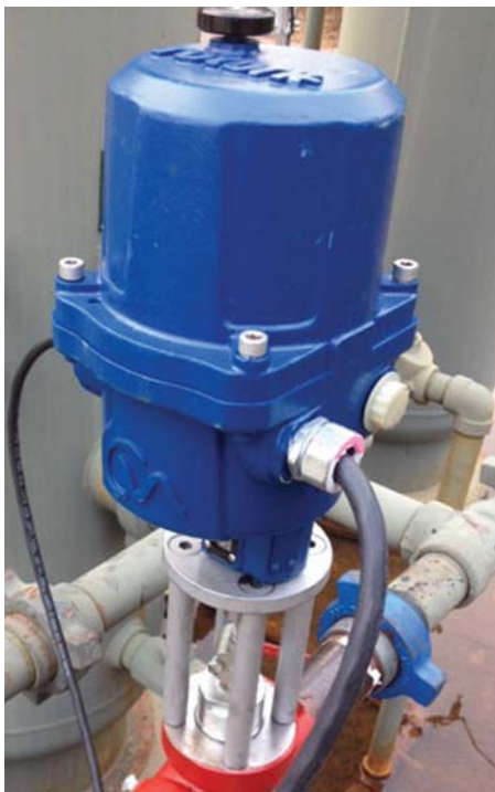
Fig 2 – Retrofit installation of Rotork CMA electric actuator on a high pressure control valve at a shale gas well in Louisiana.
