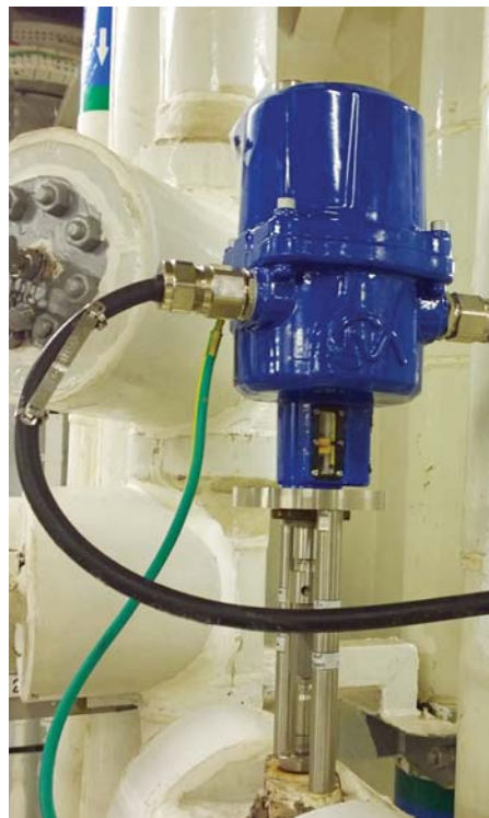
Fig 3 – Rotork CMA actuator installed on the HVAC system of an FPSO.
