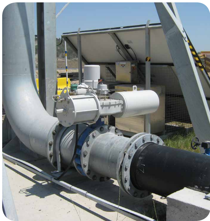
The Rotork Skilmatic Pro electro-hydraulic valve actuator installed on the Water Cart Fill Point. Solar panels seen in the background provide the renewable energy source to operate the actuator.
