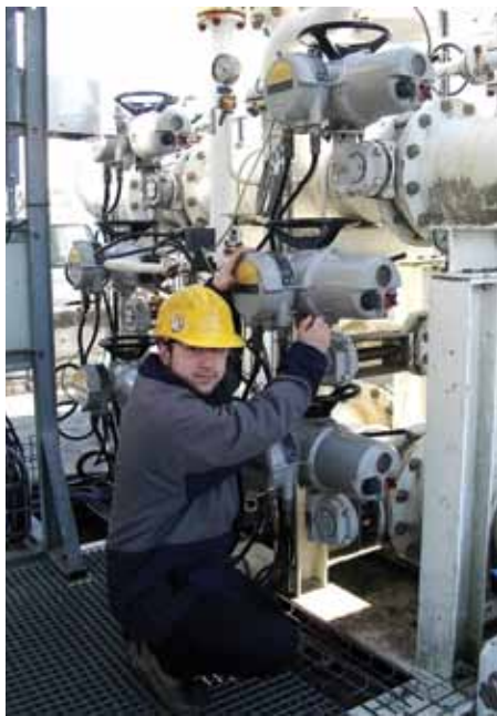
Rotork IQPro intelligent electric valve actuators on a vapour recovery unit at a refinery.
