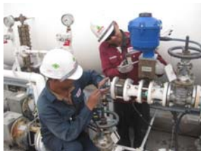
Fuel Gas Control - Thailand
