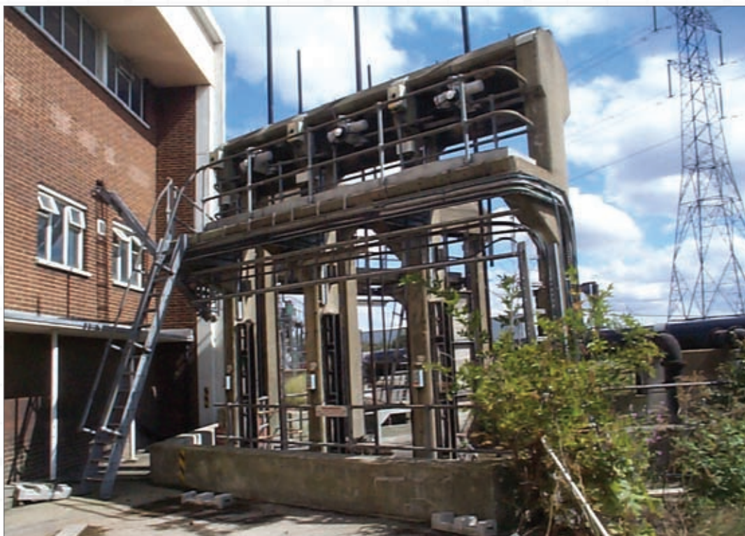
Beckton STW inlet penstocks upgraded with Rotork IQ actuators
