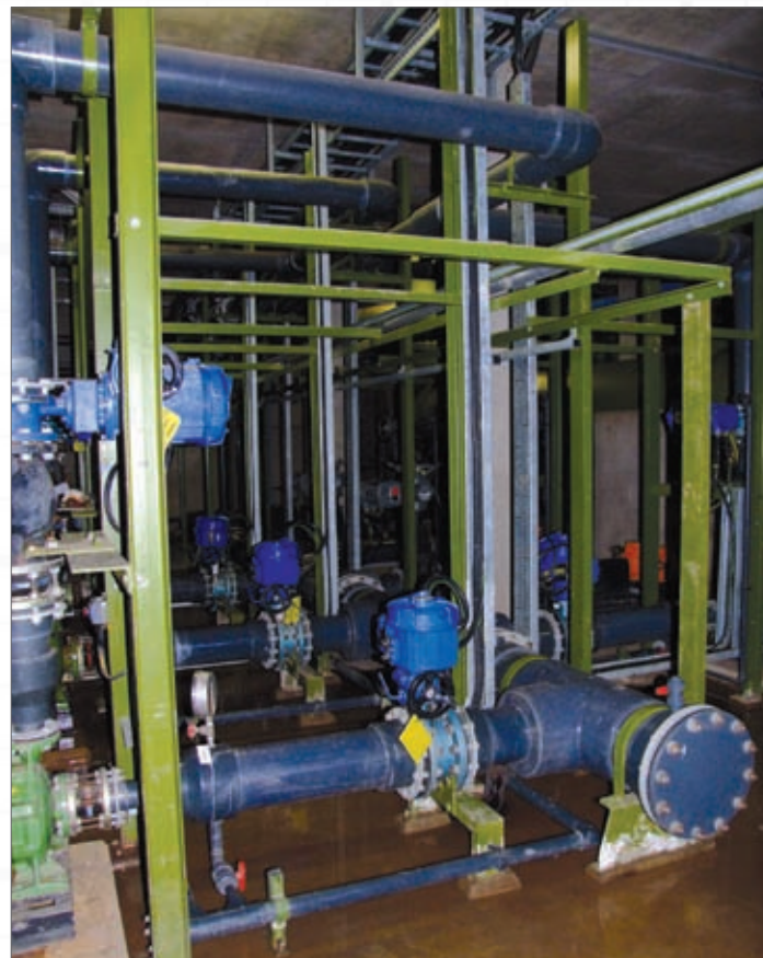
AQ and A range actuators in the rapid gravity filter plant. The flood water level here reached above the ceiling of the chamber
