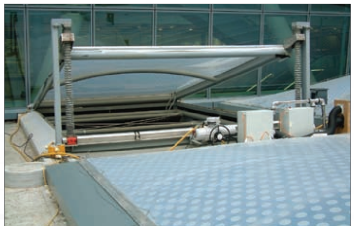
IQ actuator installation in progress on one of the T5 fire doors
