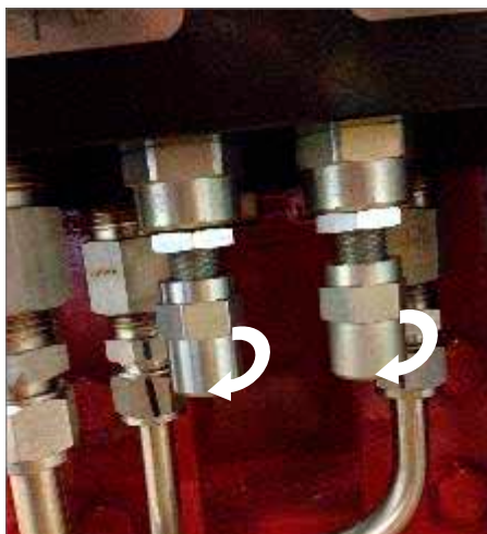
Fig 12.6 Flow regulator cap removal
