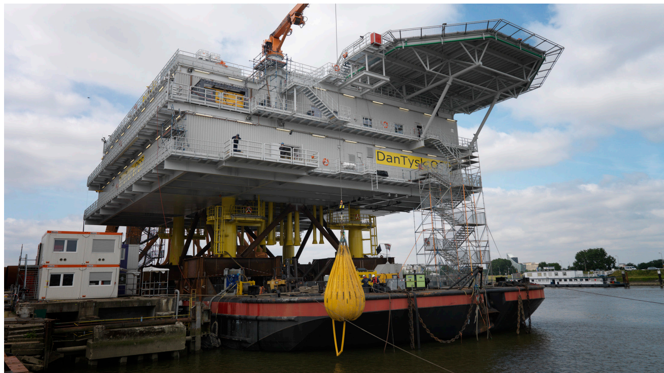
Above: The DanTysk offshore wind farm substation being prepared for its final destination off the island of Sylt in the North Sea.
