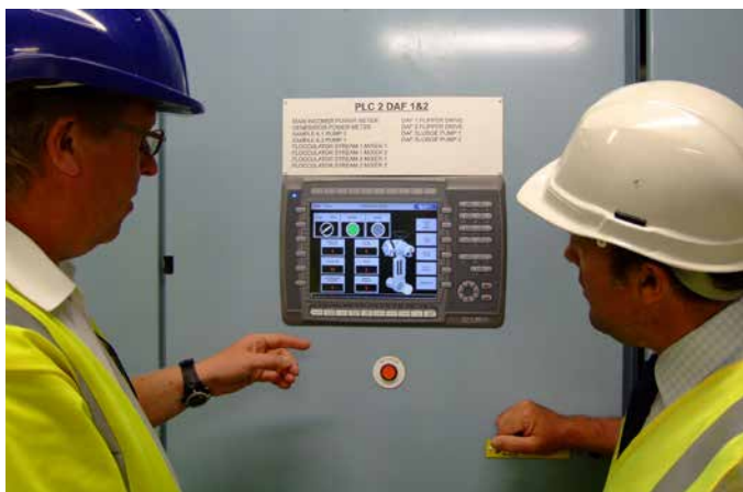
HMI screen at Maundown. The Rotork actuators can be interrogated, monitored and controlled at these stations.
