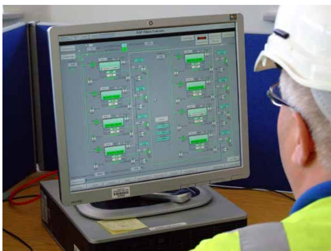
SCADA screen at Maundown, monitoring the operation of rapid gravity filters.
