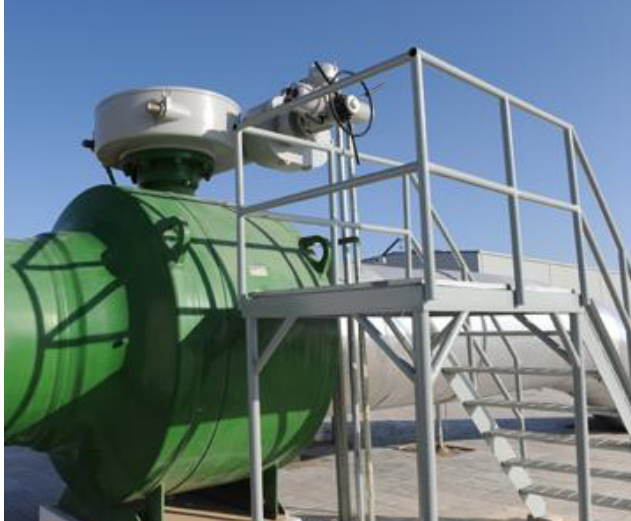
IQ actuator with gearbox installed on one of the pipelines.
