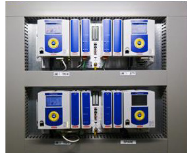
Pakscan Master Stations monitoring and controlling the IQ and Skilmatic SI actuators at BTT on three separate bus networks. Designed specifically for the valve actuation environment, Pakscan incorporates secure field communications with inbuilt network redundancy to maintain control even in the event of equipment or cable failure.
