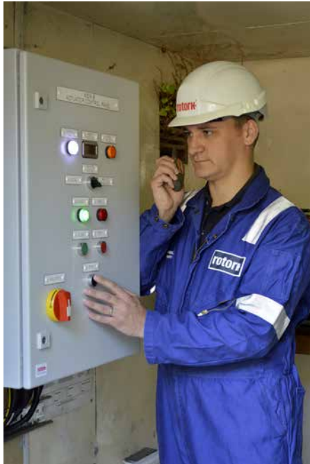
A Rotork engineer confirms the successful operation of the new control panel during site commissioning.
