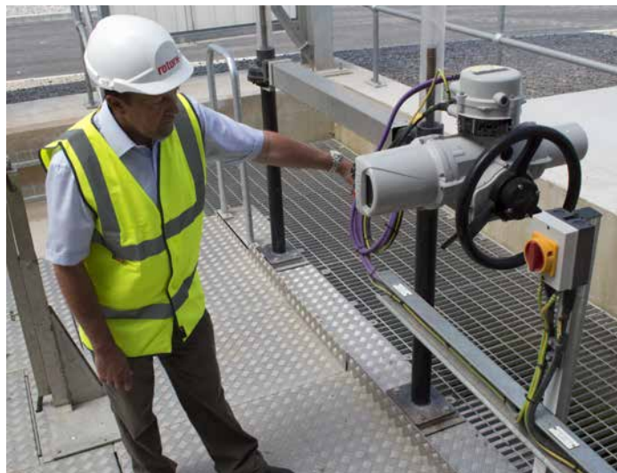
This IQ3 unit, the latest version of Rotork's intelligent actuation product range, drives through Rotork IB gearboxes and extension drive shafts to control the position of the two outlet modulating penstocks on the site's new Ultra-Violet disinfection plant.
