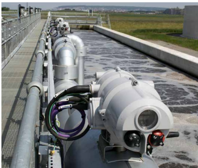
Profibus-DP V1 enabled Rotork IQT intelligent electric valve actuators control the air supply to the new activated sludge plant (ASP) at Weston-super-Mare STW.
