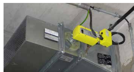
Schischek ExMax actuator installation on one of the air dampers.
