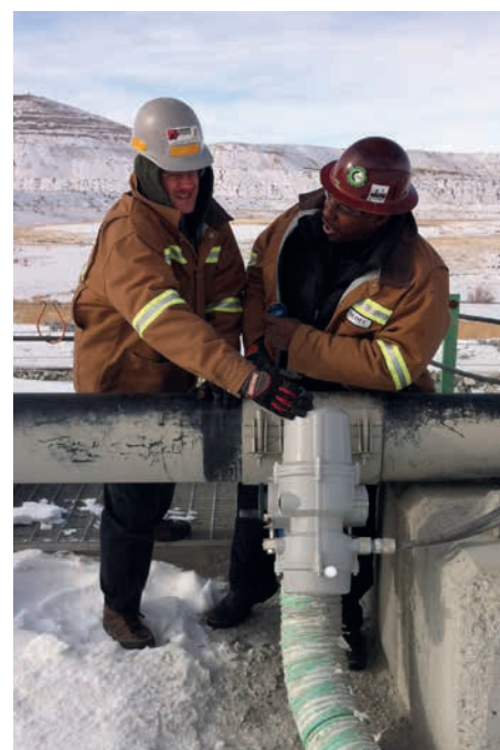
James Hall and Mark Dennis from Rotork's service team complete the non-intrusive commissioning of one of the 12 Rotork IQT actuators that control the flow of water into the filter bags.
