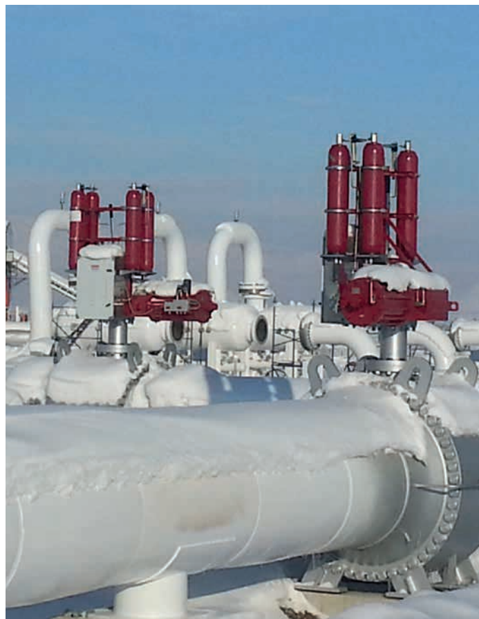
Rotork GO Range gas-over-oil valve actuator installations at the Erzincan compressor station.
