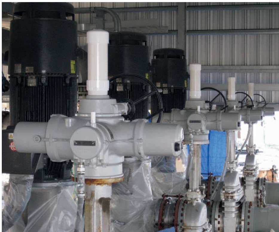
Rotork IQ40 actuators installed on the four booster pumps, again illustrating the simplified site wiring. Note the wireless Pakscan antennas on each actuator's terminal housing.
