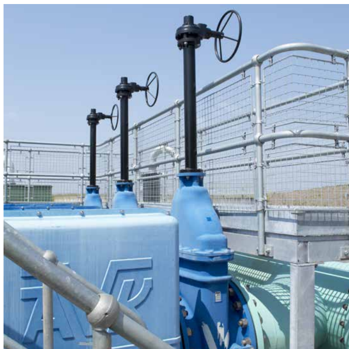
Rotork IB gearboxes are installed for the manual operation of isolating valves at site locations including the pumping stations.
