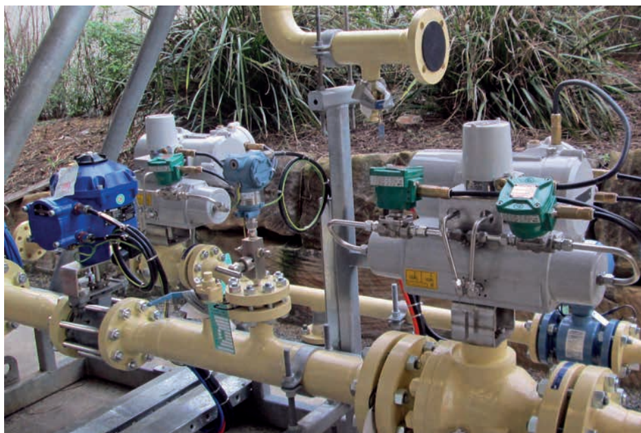
Rotork CVA and Skilmatic actuators installed on a typical Queensland Gas wellhead skid. On the left, a CVA actuator, model CVQ1200, operates a 3 inch (DN80) ball valve to control the gas flow and pressure. Behind the CVA, a Skilmatic Model SI-Q51 electro-hydraulic actuator operates a 2 inch (DN50) safety shutdown ball valve on the water extraction line. The Skilmatic Model SI-Q60 on the right is controlling a 4 inch (DN100) safety shutdown ball valve on the gas line.
