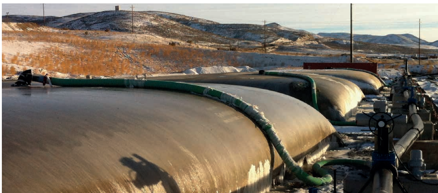
A section of the Geotube® dewatering plant, with the Rotork IQ actuators installed on the inlet pipework on the right hand side. In total there are 12 filter bags, of which 3 can be seen in this view below.
