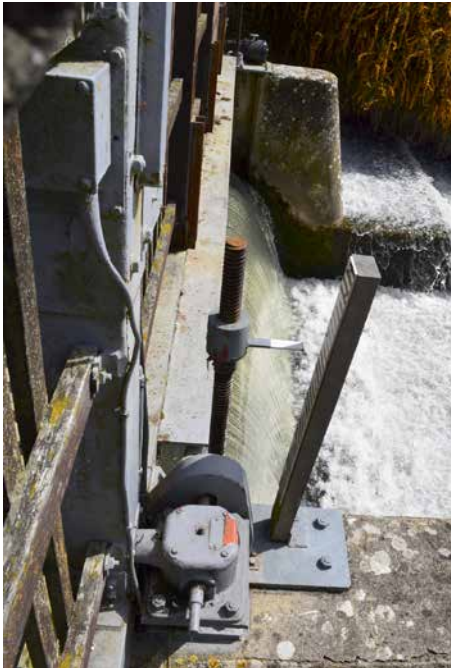
Close-up of the obsolete sluice gate motor drives.
