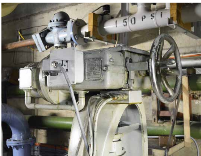
One of the original Rotork 100A valve actuator installations.
