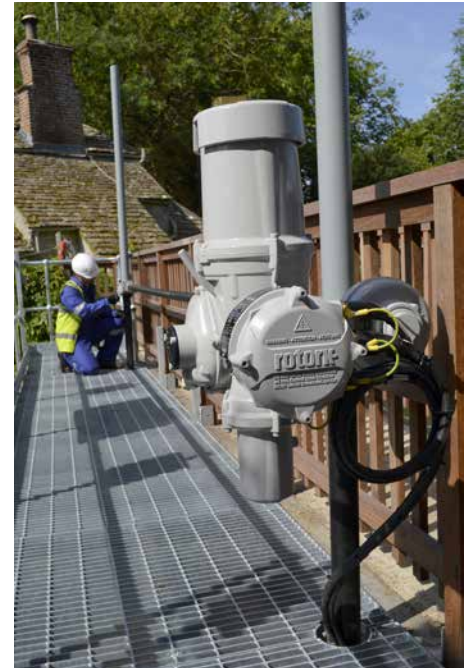
Installation nearing completion on the new walkway platform; the IQ3 actuator in the foreground is fitted with its vandal-proof cover.
