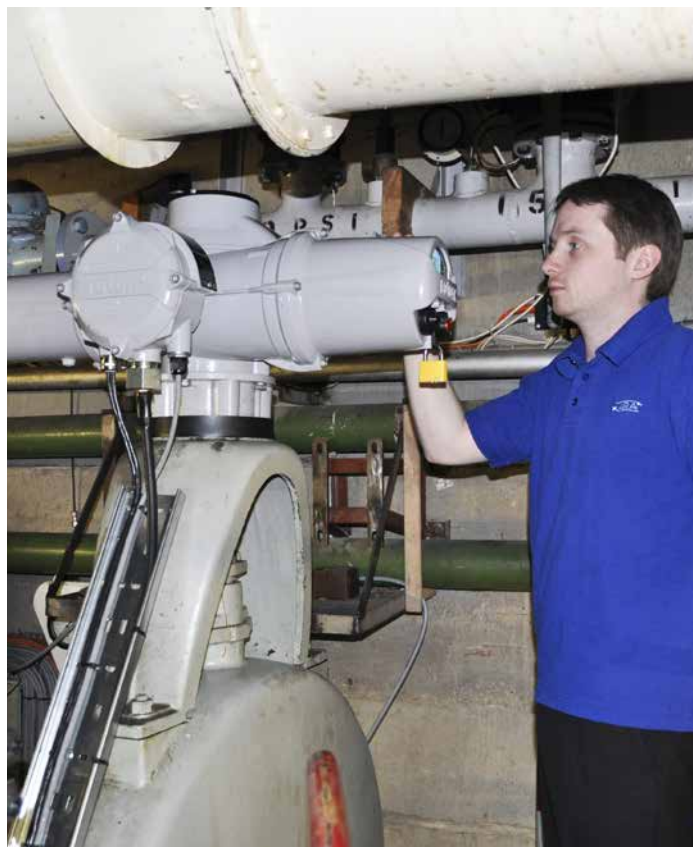
Richard Harvey, Senior Process Engineer at the Aircraft Research Association, inspects the same valve, now retrofitted with a new Rotork IQ3M actuator.
