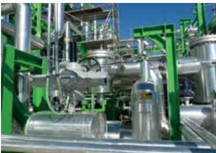
The actuators provide increased efficiency at solar plants
