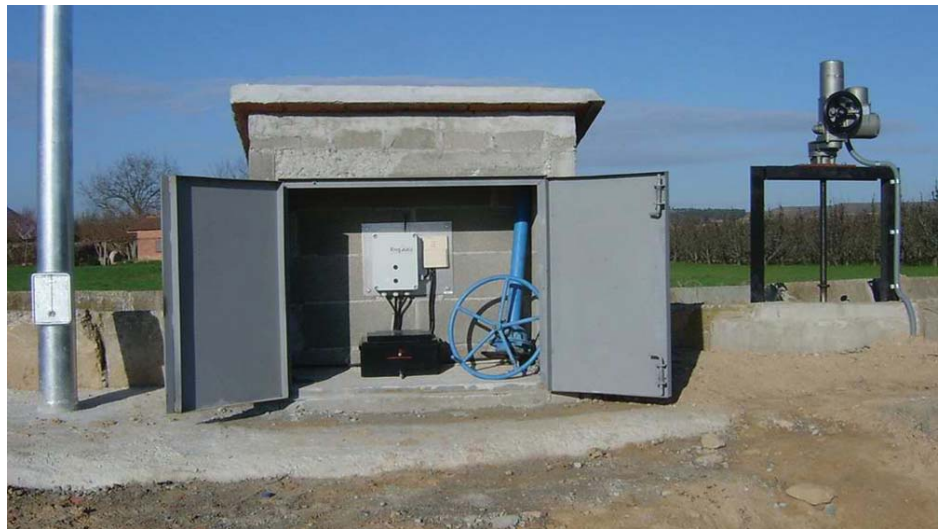
A retrofitted solar powered low voltage installation, with a Centork DC actuator fitted to an existing penstock, replacing the original handwheel awaiting disposal in the new control cabinet.
