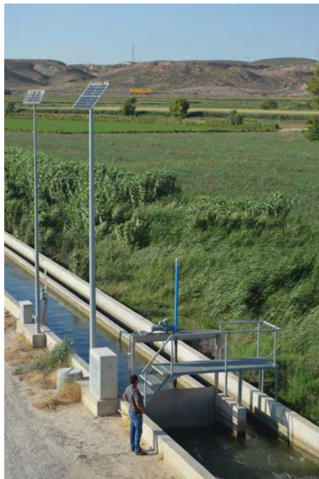
Typical solar powered remote penstock installations equipped with 24VDC Centork actuators. (Photo courtesy of Riegosalz)
