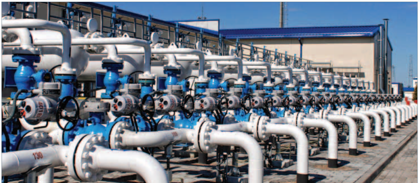
Rotork IQ intelligent electric valve actuators installed on the gas injection plant at Incukalns.
