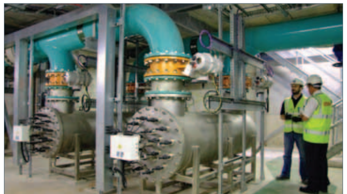
The state-of-the-art, low pressure Ultra Violet disinfection plant installed at Cwellyn.
