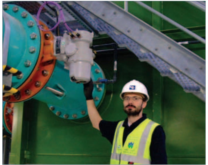
Rotork IQTM modulating actuator controlling a steady flow of water into the DAF plant during the flushing operation, when the water level in the filter is raised to enable floating effluent to escape over a weir.
