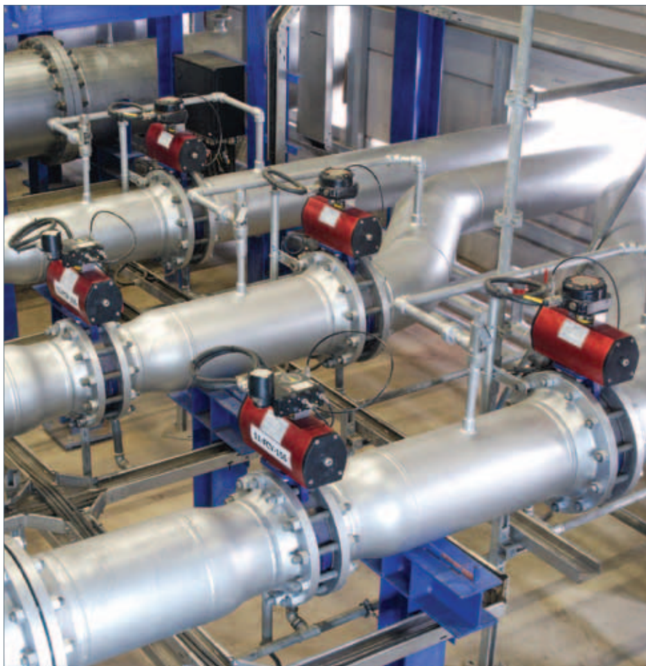
Some of the Rotork RC200 Series pneumatic valve actuator installations on the liquid meter calibration loop at EuroLoop.
