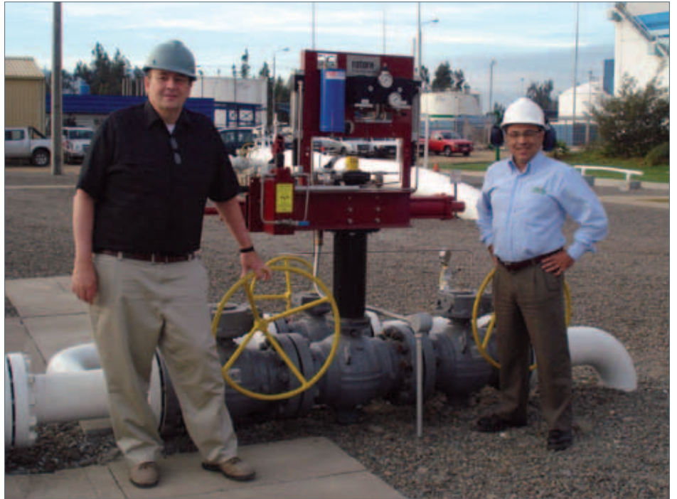
One of the Rotork HPG actuator installations at the Electrogas gas terminal in Quillota.
