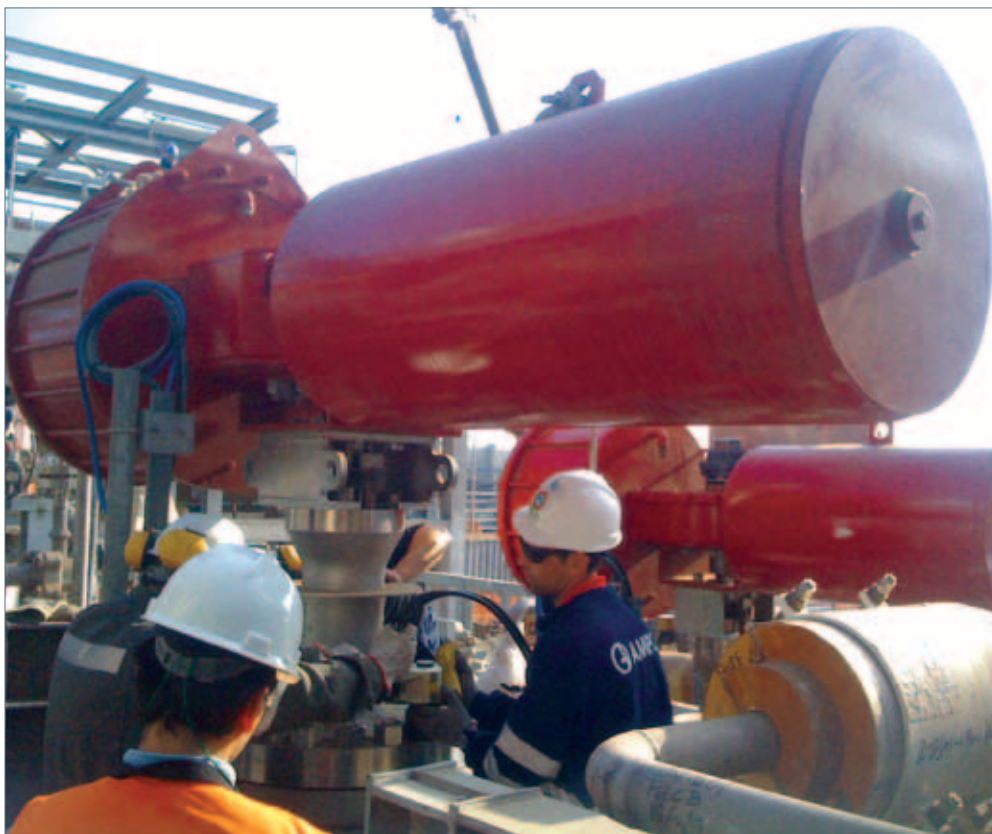
Rotork GP range, spring-return, scotch-yoke pneumatic actuator installations on the sea terminal at Quintero Bay.
