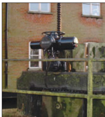
One of the completed Rotork IQ actuated sluices at Dedham Mill.
