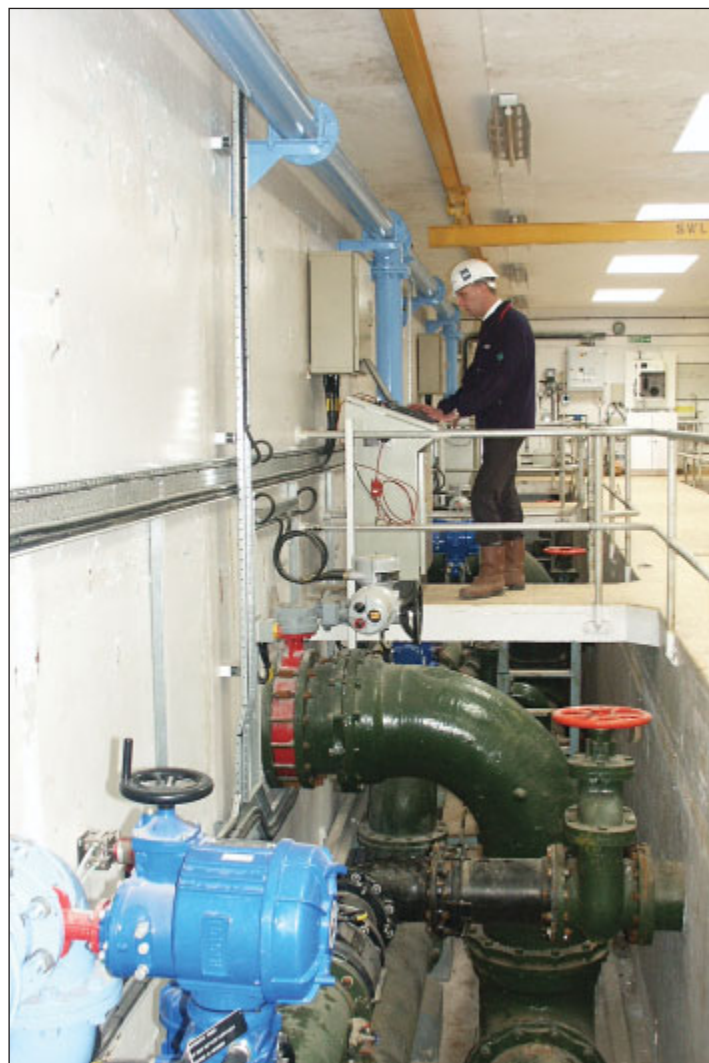
Norwest Holst M & E Supervisor Kevin Roddenby inspects a Rotork IQ actuator installed on a Bamford filter inlet penstock and (right) downloads operating data from IQ and AQ actuators installed on backwash and air scour valves.
