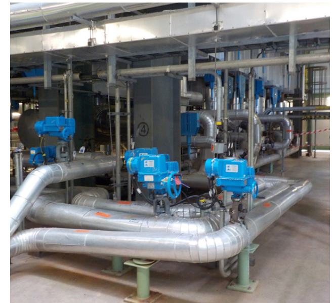
Above: An area of blowdown valves prior to the upgrade.
