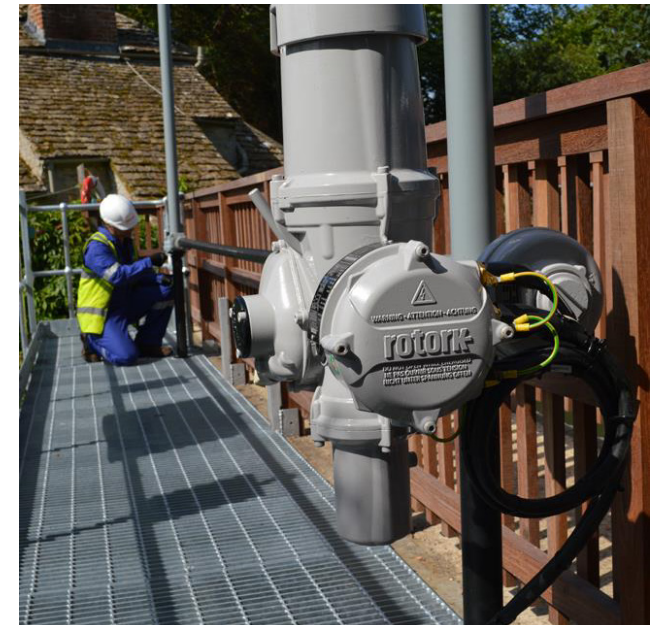
Installation nearing completion on the new walkway platform; the IQ3 actuator in the foreground is fitted with its vandal-proof cover.
