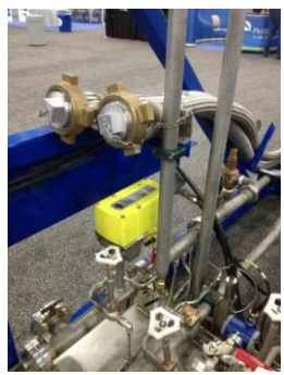
Schischeck ExMax on a process skid
