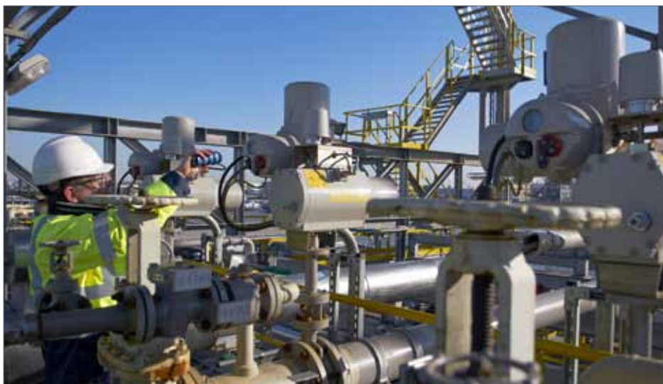
Rotork Skilmatic SI electro-hydraulic fail-safe valve actuators on the loading jetty.
