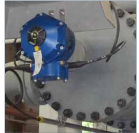
A completed CVA actuator installation on one of the pre-heater skids at the Petrogas Gas Systems factory.
