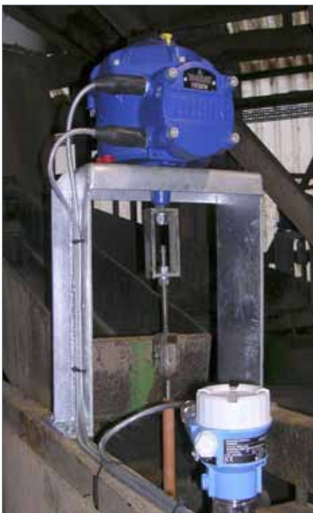
A Rotork CVA actuator installed on a TBS Hydrosizer, operated by the control signal from the adjacent density probe.
