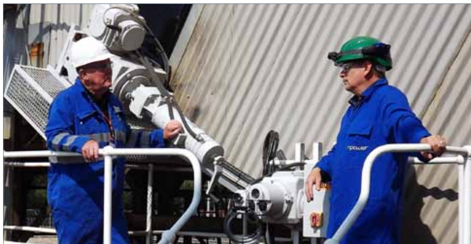
Andrew Millard (right) Control & Instrument Engineer at Fawley Power Station pictured with Mike Dale from EXEECO APS (left) by the Rotork Type SM-6000 actuator.
