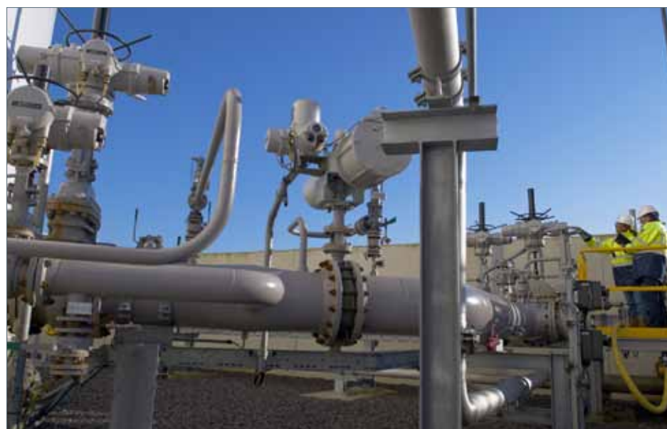
Rotork IQ Pro and Skilmatic SI valve actuators in a tank manifold area.
