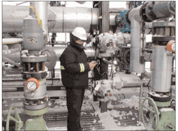
Rotork engineer Mike Joslin demonstrates the user-friendliness of non-intrusive IQ actuator commissioning in the freezing conditions of BP Borealis (above) and inspects one of the P range pneumatic actuators installed at the same site (top).
