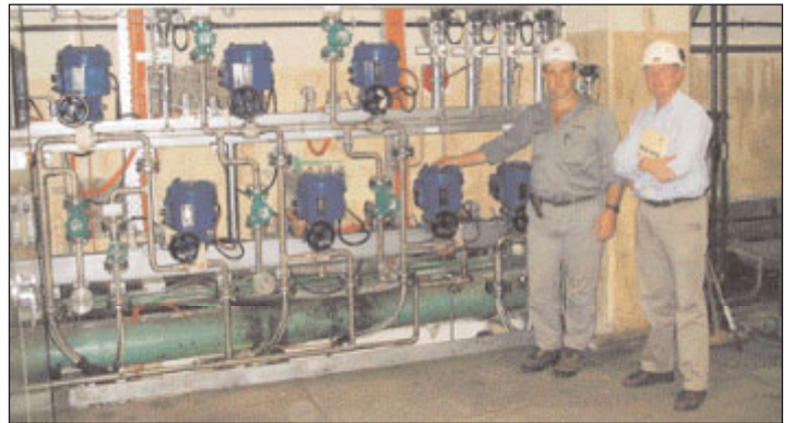
Below Trevor Downing from Stanwell Corporation and Rotork's Jeff Quarrell with seven of the newly installed AQ actuators in the generator hall at Kareeya Hydro.
