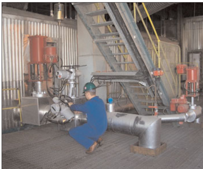
Economiser re-circulation pipework at Ratcliffe, equipped with failsafe Rotork Skilmatic SL and SHL linear and SQ quarter-turn modulating actuators, together with Rotork IQ25 and IQ12 isolating actuators.
